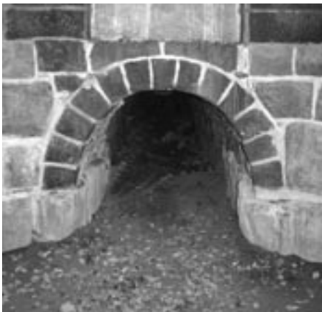
Newly restored tailrace arch in turbine chamber of Plane 2 East. Prior to the project the arch was collapsing.
